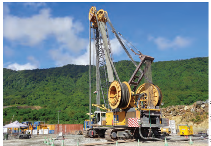
In addition to a Bauer MC 128 duty-cycle crane with BC 30 cutter unit, an MC 96 duty-cycle crane with grab and a Bauer BG 45 rig with double-walled casing have been used on this project.
