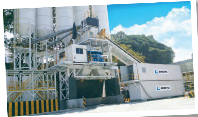
TOP AND ABOVE: The Eurotec MZ 6750Ti concrete batching plant and the flake ice plant are working in tandem to ensure the project remains on track. One of the initial tasks for the MZ 6750Ti was mixing concrete for the tower’s foundations. This required pouring 137 reinforced concrete bored piles, each measuring 60 m deep and 2.2 m in diameter.
