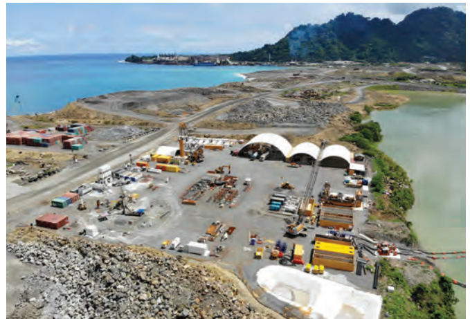
Bauer Engineering PNG Ltd executed two test cut-off wall elements up to a depth of 55 m below the ground surface.
